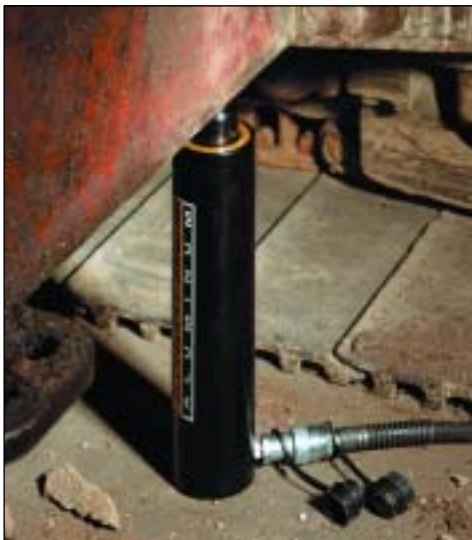
◀ A lightweight RAC-208 provides plenty of force to lift this excavator for track maintenance.
